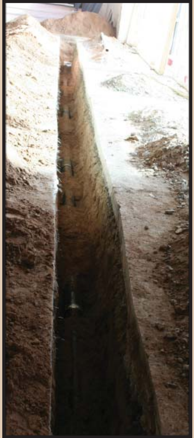
Wastewater Line, Shiprock Behavioral Health Center
